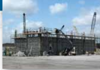
South District Treatment Plant, Miami-Dade County, Florida, USA Miami-Dade County
